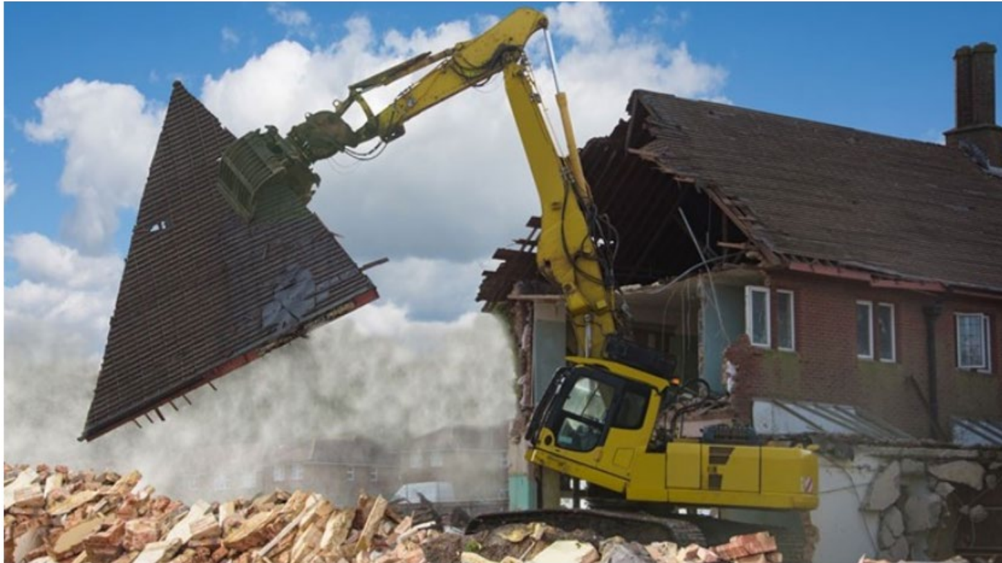
Earlier this year, crews removed roofing, flooring and walls in a project that's part of a Cornell University study comparing deconstruction and demolition.
